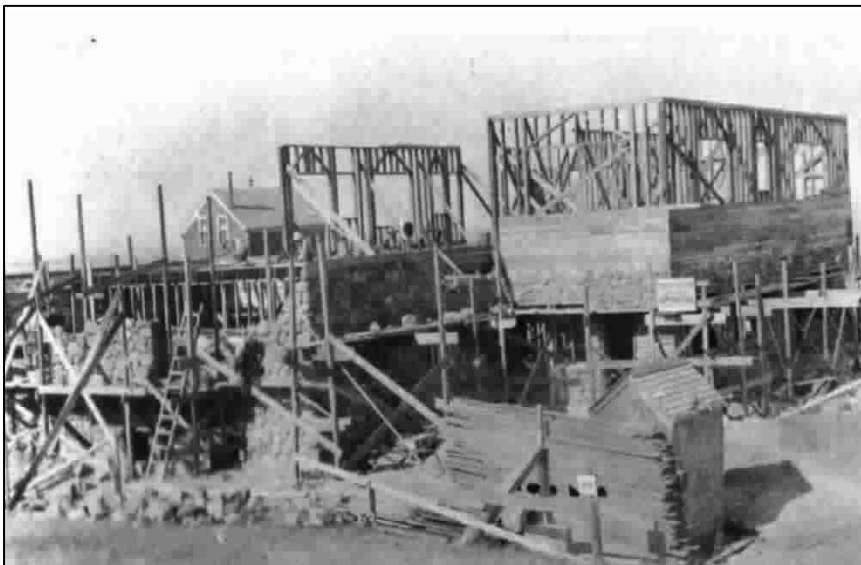
Early stage of construction of Winter House, 1916. The sign reads "Pierce and Kilburn, General contractors." CHS collection.
