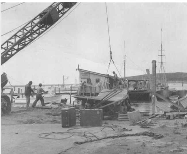
A few days later workmen assess the damage and begin repairs on the Fish Dock.
